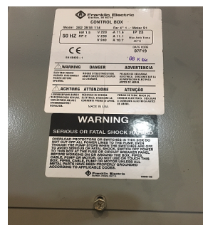
STARTER EL. ORMAR
